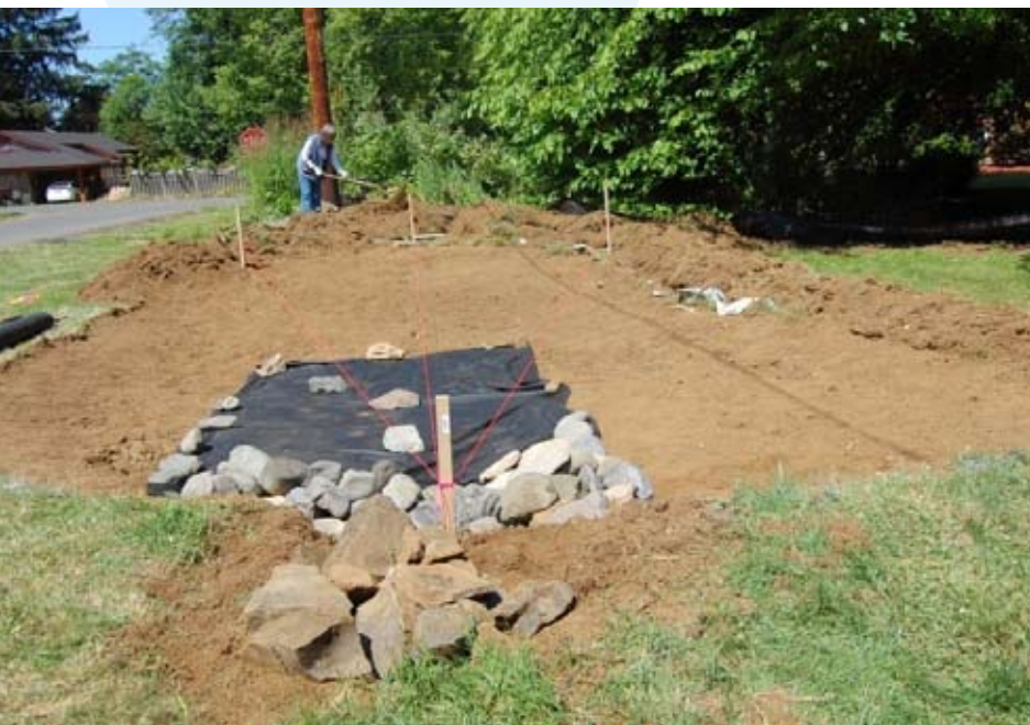
Figure 19: Grading is made simpler by using four stakes, one at the inflow point and three at the opposite or lower end of the rain garden—including, most importantly, the outflow point. (Photo: Robert Emanuel, OSU)
