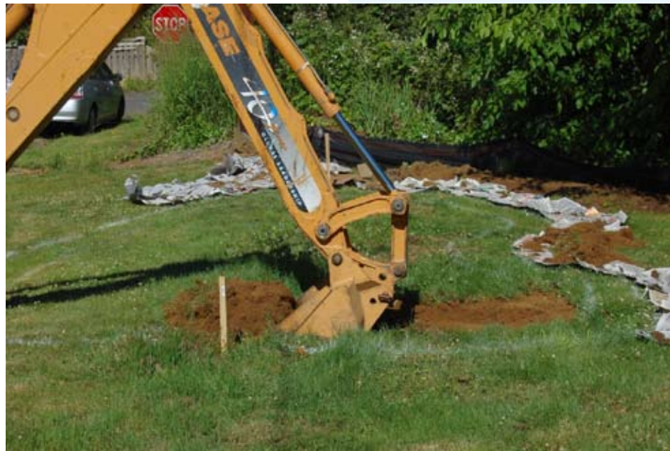
Figure 18: Excavator is located outside of the rain garden to remove soil to make sure the machine does not compact soil in the rain garden.
