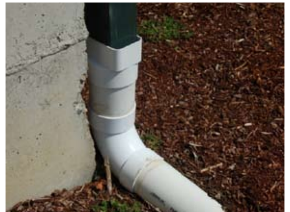
Figure 21: Four-inch ABS storm-drain pipe connects smoothly to a downspout from a roof to a rain garden in Pacific City, Oregon. (Photo: Robert Emanuel, OSU)
