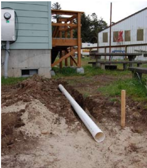
Figure 22: Four-inch ABS pipes here will convey water from this building into a rain garden. Pipes like these must be graded to drop about 1 inch for every 10 feet so that water flows away from the building but does not build up too much velocity by the time it arrives in the rain garden. (Photo: Robert Emanuel, OSU)
