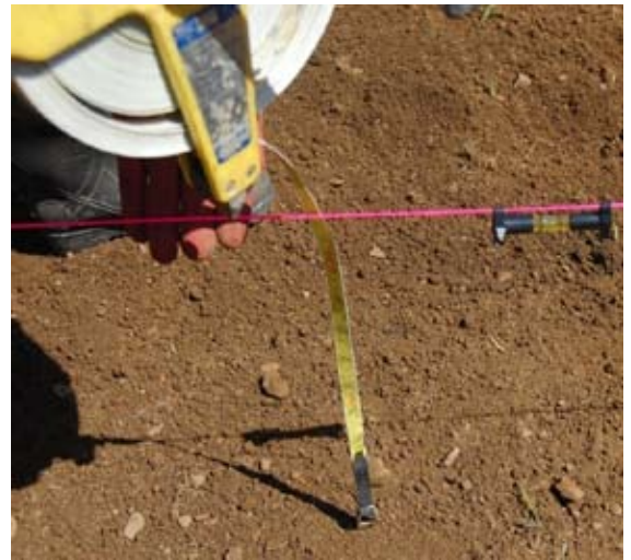
Figure 20: Using a combination of a line level and a measuring tape allows you to grade the base of the garden so that water will not pool in a particular location but will spread across the entire surface as evenly as possible. (Photo: Robert Emanuel, OSU)
