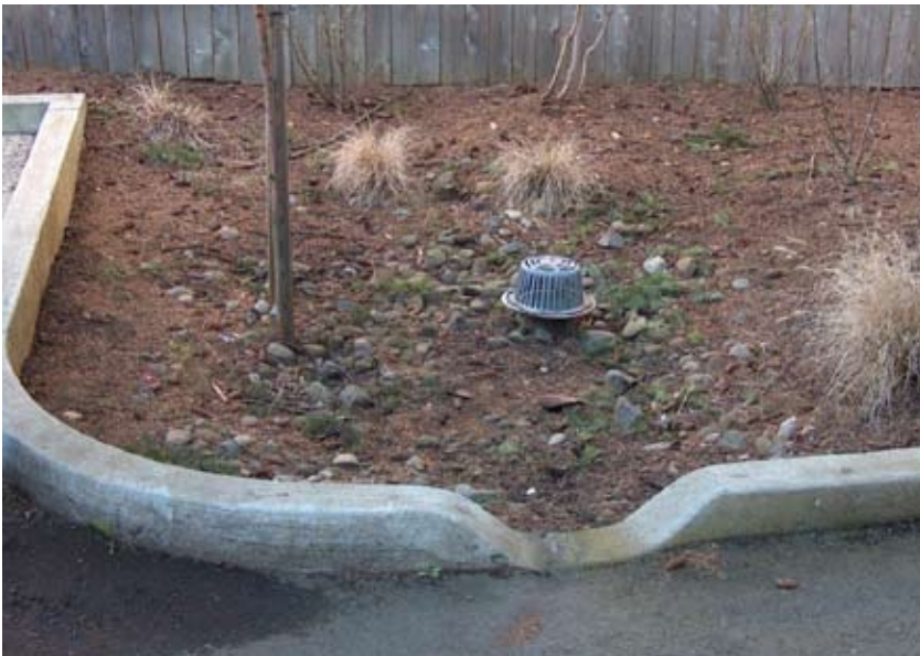
Figure 15: Curb-cut inlet for a parking lot and an overflow device (pipe and screen) for a parking lot in Gresham, Oregon. (Photo: Derek Godwin, OSU)
